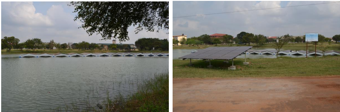
Figure 1: Floating Solar Plant at Killinochchi Premises of the University of Jaffna
